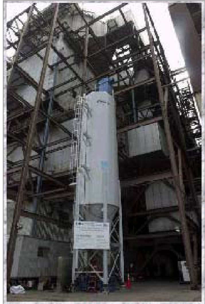
Activated carbon storage and feed system
