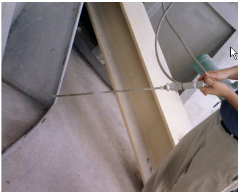
Figure 8-9. Suwannee American Cement ammonia injection nozzle.
