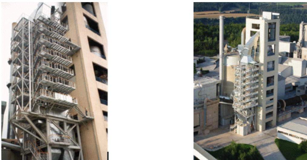
Figure 10-1. SCR system adjacent to preheater tower at Solnhofen Portland cement plant. 5
