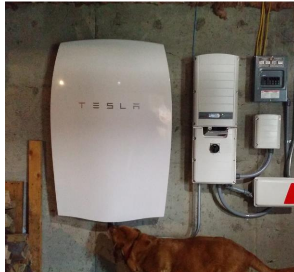
On-site generation and storage can ensure service during an outage
