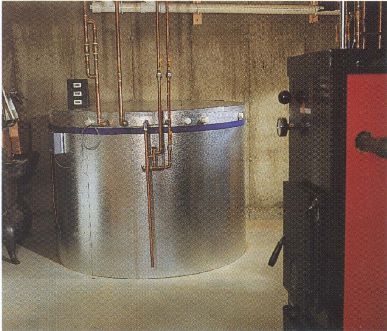
BAXI/HS-TARM boiler with Heat Storage System.
