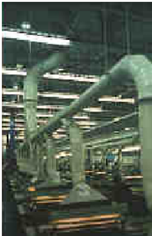
Figure 3-14. Stationary hood in an industrial process
